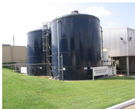
Figure 3: Effluent Treatment Plant at GGBL in Kumasi (Kaasi)
