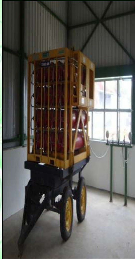
Cylinder Cascade for bottled biogas
