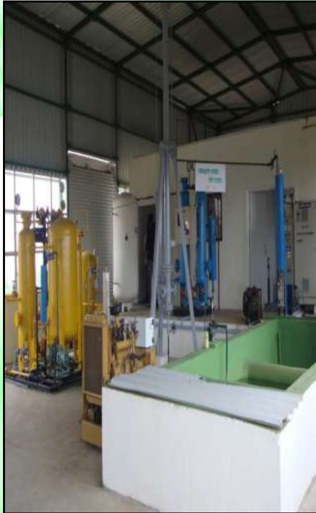
Water Scrubbing and PSA system at Nasik
