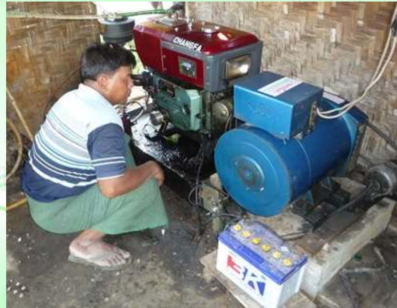
Biogas Engine for electricity production
