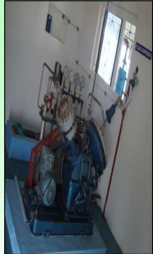
High Pressure Compressor at Nasik plant
