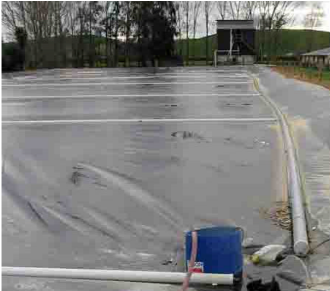
Covered Anaerobic Pond showing layout of weight pipes and rainwater pump
