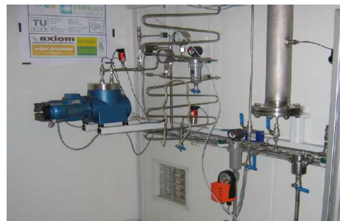
Installation of membrane to purify agricultural biogas.
