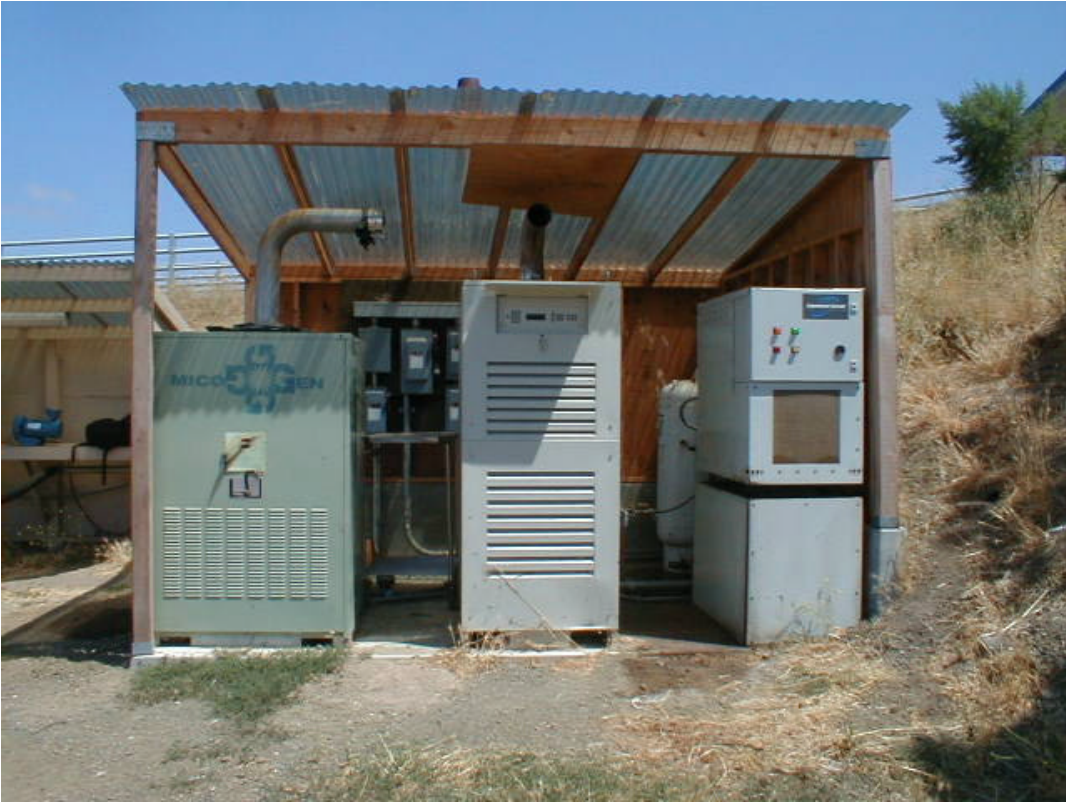
Figure 1. Microturbine Electric Generator System and Covered Lagoon Digester System
