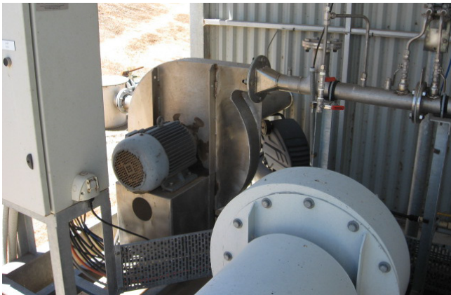
Biogas blower and flow meter. Photo courtesy of GWF Bears Lagoon Piggery
