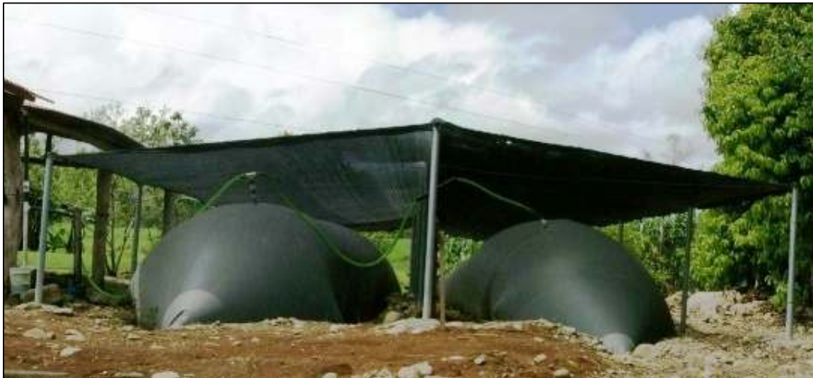
Figure 1. Biogas system; Tubular PVC membrane bags.
