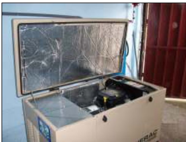
Figure 3. Biogas engine generator unit
